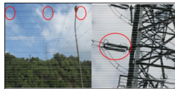
Fig. 1. Three OHGW and 22 pieces porcelain insulator
